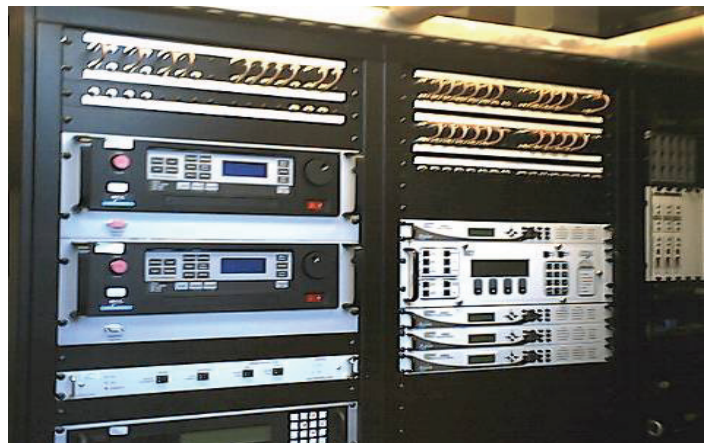
A large, rack-mounted baseband package such as this one housed in a DKET shelter, can deliver the performance needed to drive major hubs and command control facilities.
